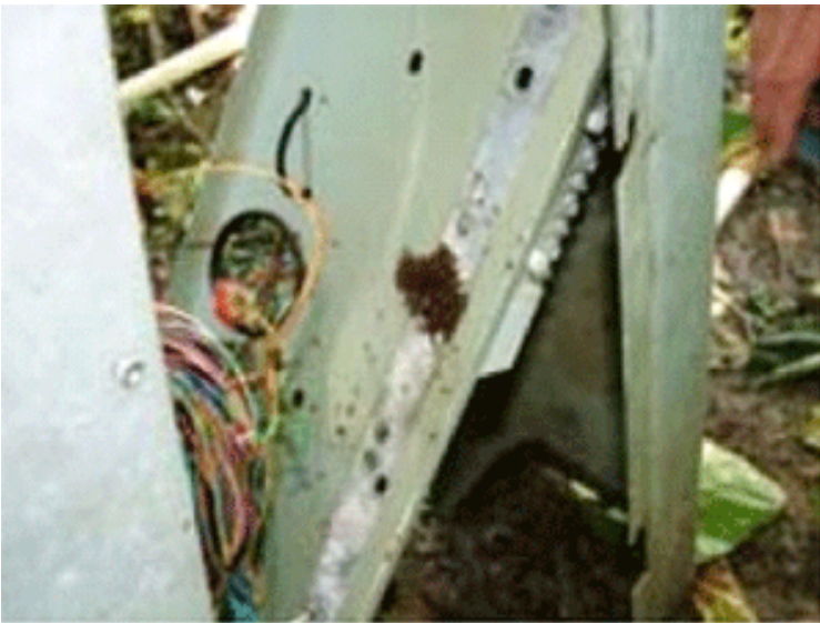
Large numbers of tawny crazy ants have accumulated in electrical equipment, causing short circuits and clogging switching mechanisms, resulting in equipment failure.
